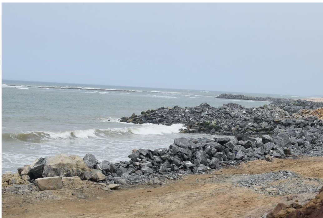
Figure 9: An image of Coastal defense structure in Ningo experiencing toe failure.
